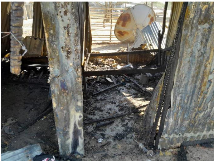
Figure 2: Destroyed Obama Inn by the fire.
